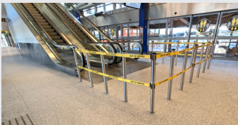
Going up? Going Down? Either way safety is top priority.
